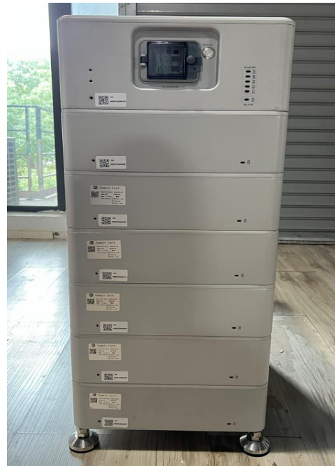
Figure 4: Side View of BESS unit
