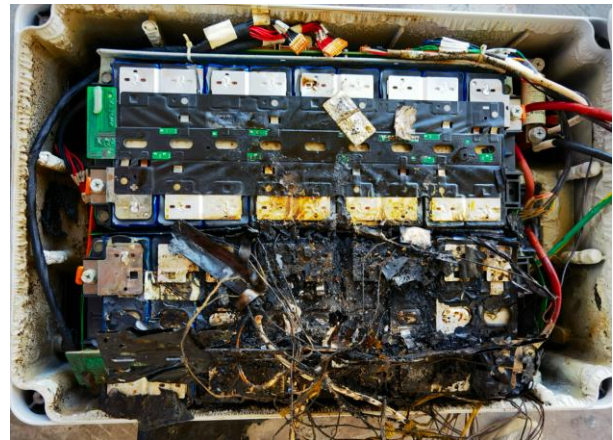
Figure 21: Internal view of initiating module
